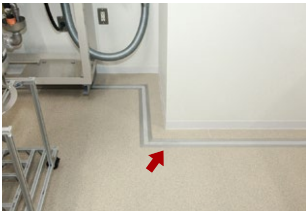
Foundation of the calibration lab is structurally separated from the skeleton of the new laboratory building, making it difficult for vibrations to be transmitted directly into the calibration lab. Silicone rubber is embedded in the gaps to ensure safety.
