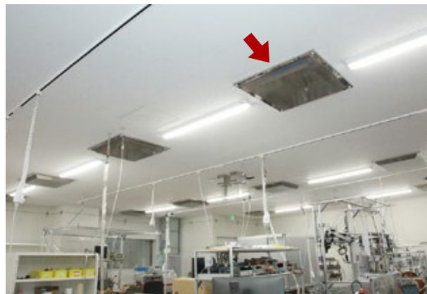
A cover (perforated metal) with small holes covering the entire surface is installed so that air from the air conditioner does not concentrate in a small area.
